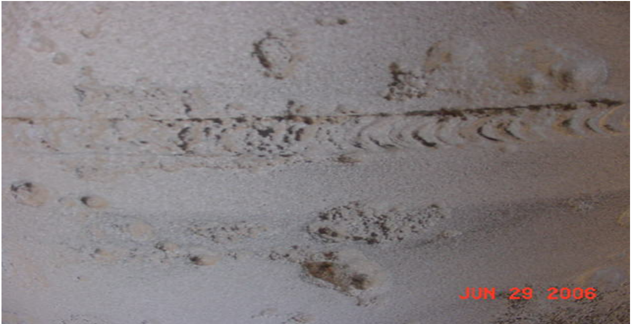
Photo #4 - Shrink sleeve applied in 1997 and resulting corrosion found in 2006. Shrink sleeve shielded the CP. Pipe potentials met all NACE criteria.
