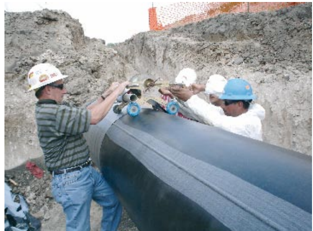
Figure 3. Field application of the RD-6 coating system on a 30 in. rehabilitation project in South Texas.
