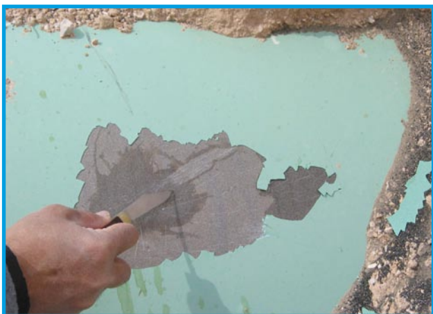
Figure 2. Even though blisters and poor adhesion were a problem, the steel under the FBE coating shows to be in excellent condition, proving 'fail safe' properties.
