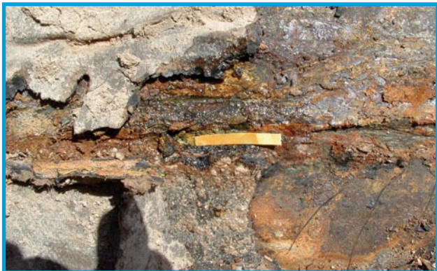
Figure 1. pH of 5 under disbonded coal tar coating with significant corrosion present (not 'fail safe').
